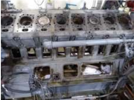
Cogenerator apart after failure
