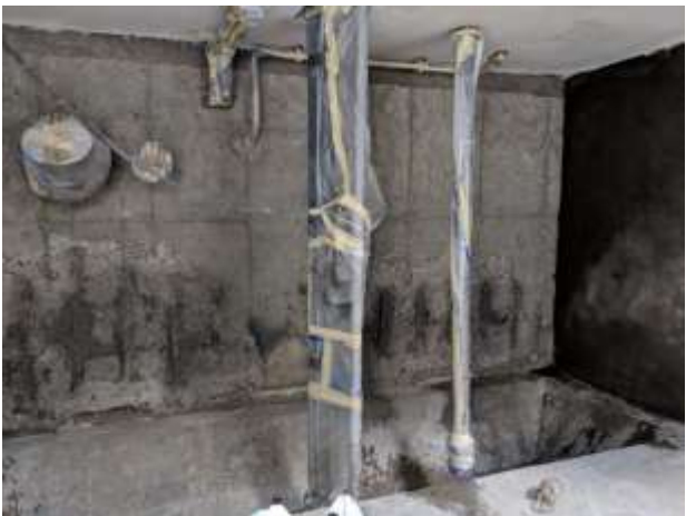
Spalled concrete in the hypochlorite drain vault
