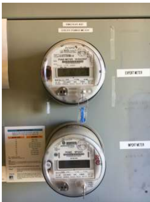
New power export meter (top)
