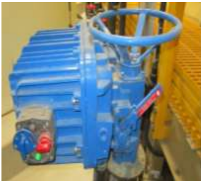
Original motorized valve operator
