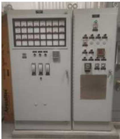
Existing control panel
