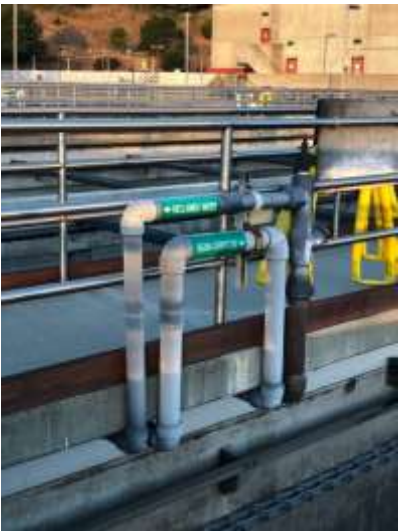
Original reclaimed water piping
