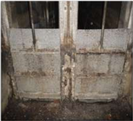
Originally installed isolation gates
