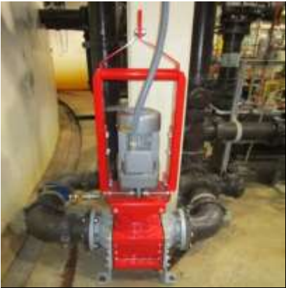
Sludge grinder cartridge and piping
