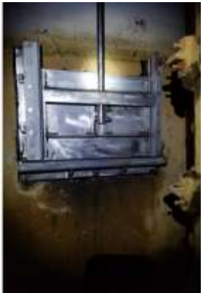
New stainless steel isolation gate
