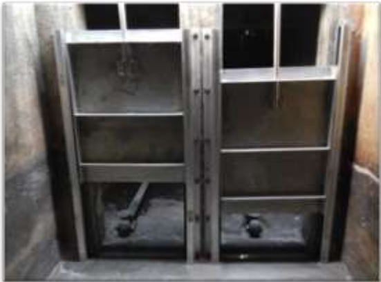
New isolation gates
