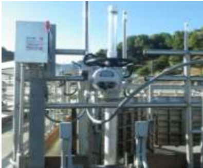
New motor operated valve
